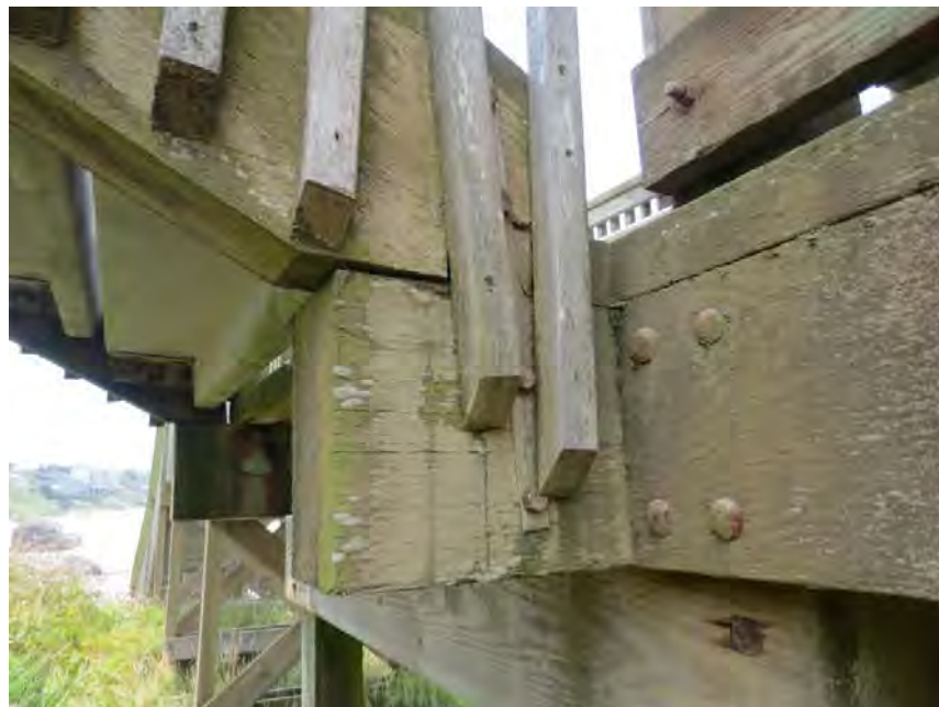
Photo 6 – Lateral Displacement at Stair to Landing Connection
