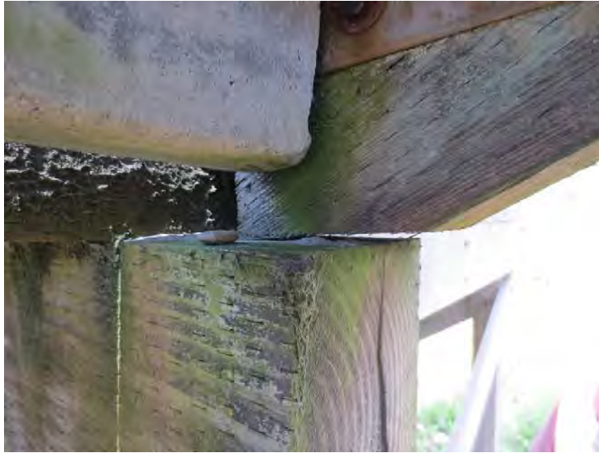
Photo 5 – Open Gap at Displaced Stair Stringer
