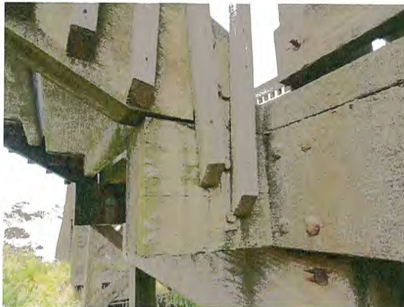
Photo 6 – Lateral Displacement at Stair to Landing Connection
