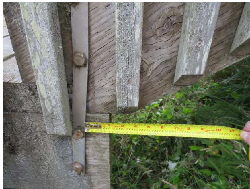
Photo 4 – Movement at Stair Stringer to Landing Connection
