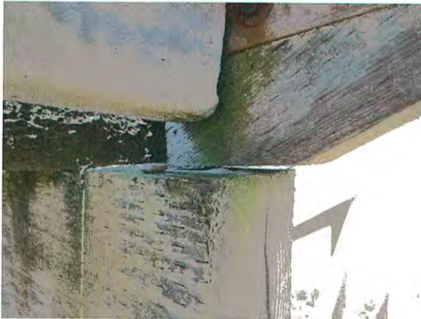
Photo 5 – Open Gap at Displaced Stair Stringer
