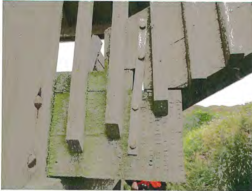
Photo 3 – Typical Movement at Stair Stringer to Landing Connection
