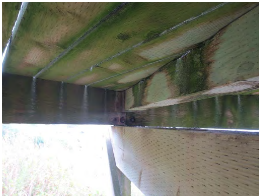
Photo 8 – Moss/Algae Growth Under Wood Decking
