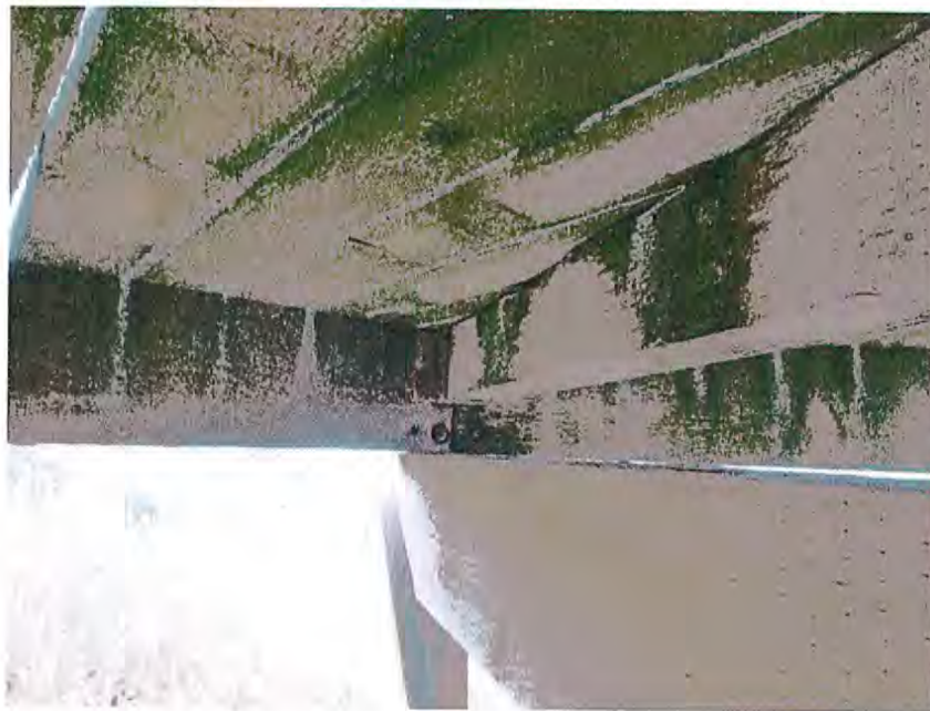
Photo 8 – Moss/Algae Growth Ender Wood Decking
