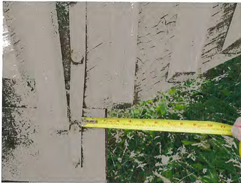
Photo 4 – Movement at Stair Stringer to Landing Connection
