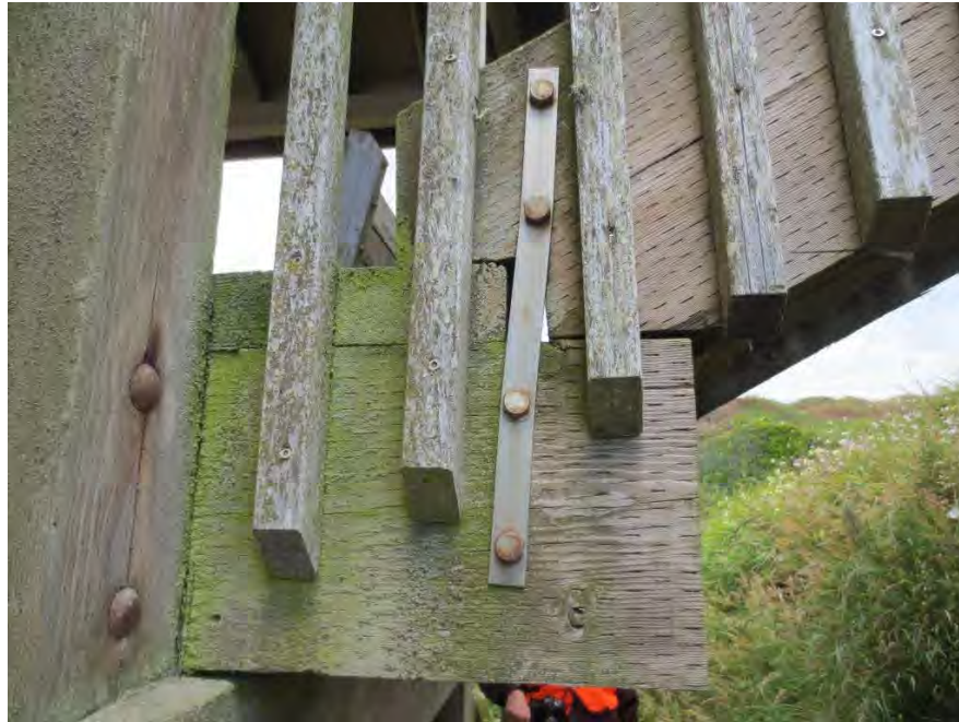
Photo 3 – Typical Movement at Stair Stringer to Landing Connection
