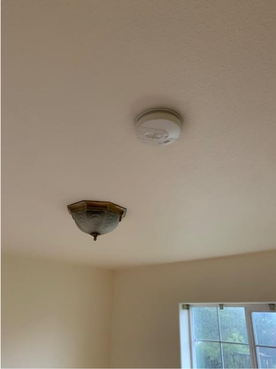
Smoke alarm in bedroom #1
