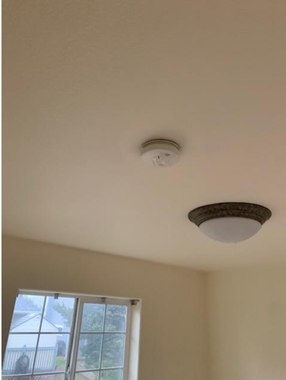
Smoke alarm in bedroom #2
