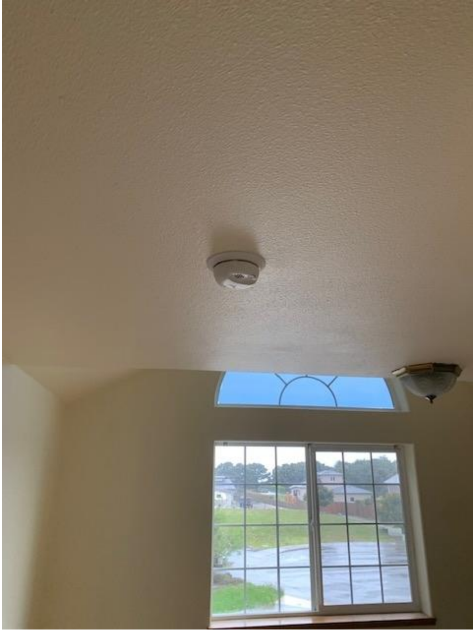
Smoke alarm in master bedroom
