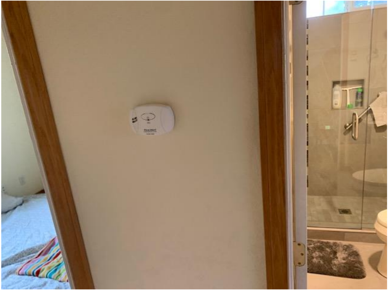
Upstairs carbon monoxide alarm
