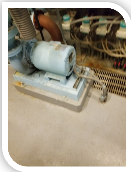
FIGURE 5.3.8 TREATED WATER PUMP
