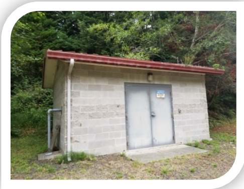
FIGURE 5.2.2 LOWER PUMP STATION
