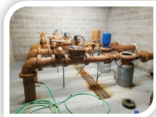
FIGURE 5.2.3 MIDDLE POND PUMP STATION
