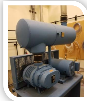
FIGURE 5.3.5 AIR SCOUR BLOWER
