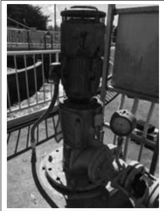
Moderate corrosion to pump motor
