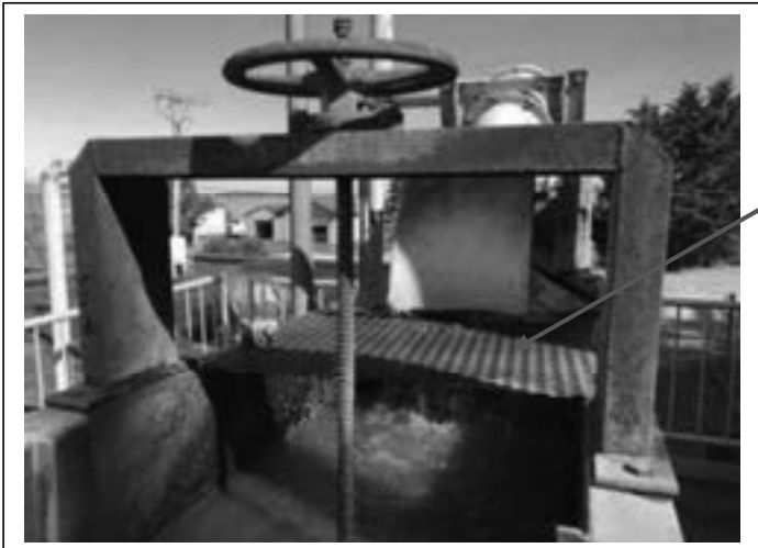
Grit Classifier shows moderate to severe corrosion throughout internal and external components. Hand operated weir is corroded in place and not operable.
