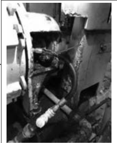
Moderate corrosion in stuffing box area.
