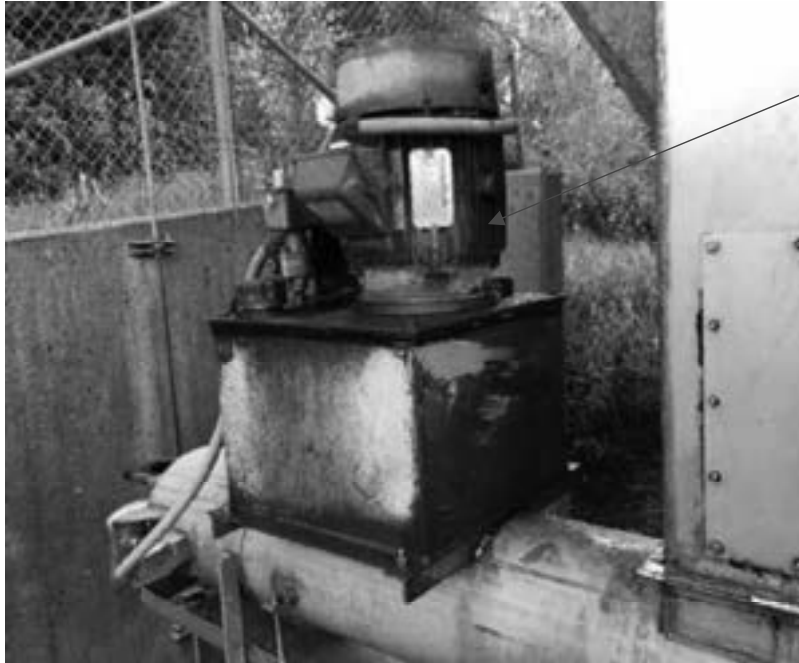
Screenings compactor hydraulic drive unit.
