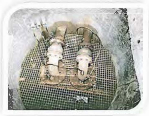
FIGURE 5.2.1 LOW FLOW PUMP STATION
