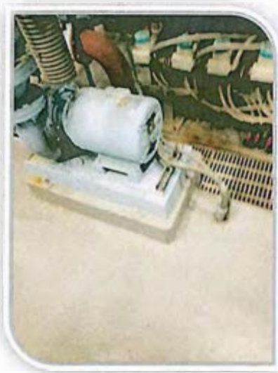
FIGURE 5.3.8 TREATED WATER PUMP
