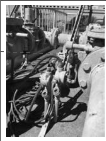
Plant drain piping manifold check valve spring severely corroded. Common to both valves.
