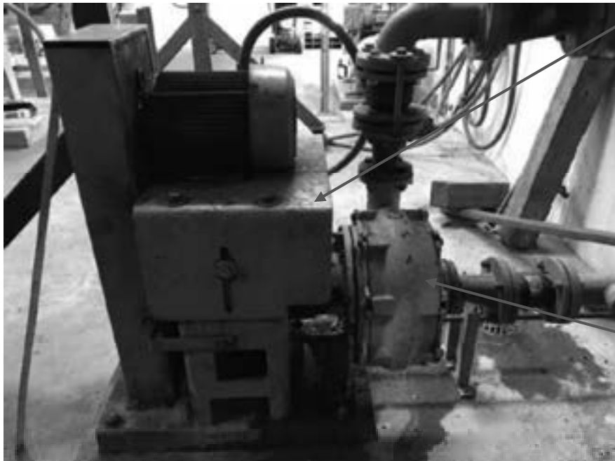
Grit Pump assembly
