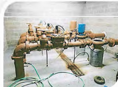
FIGURE 5.2.3 MIDDLE POND PUMP STATION
