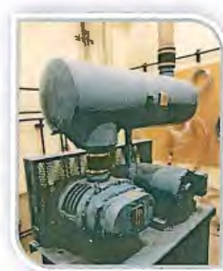
FIGURE 5.3.5 AIR SCOUR BLOWER
