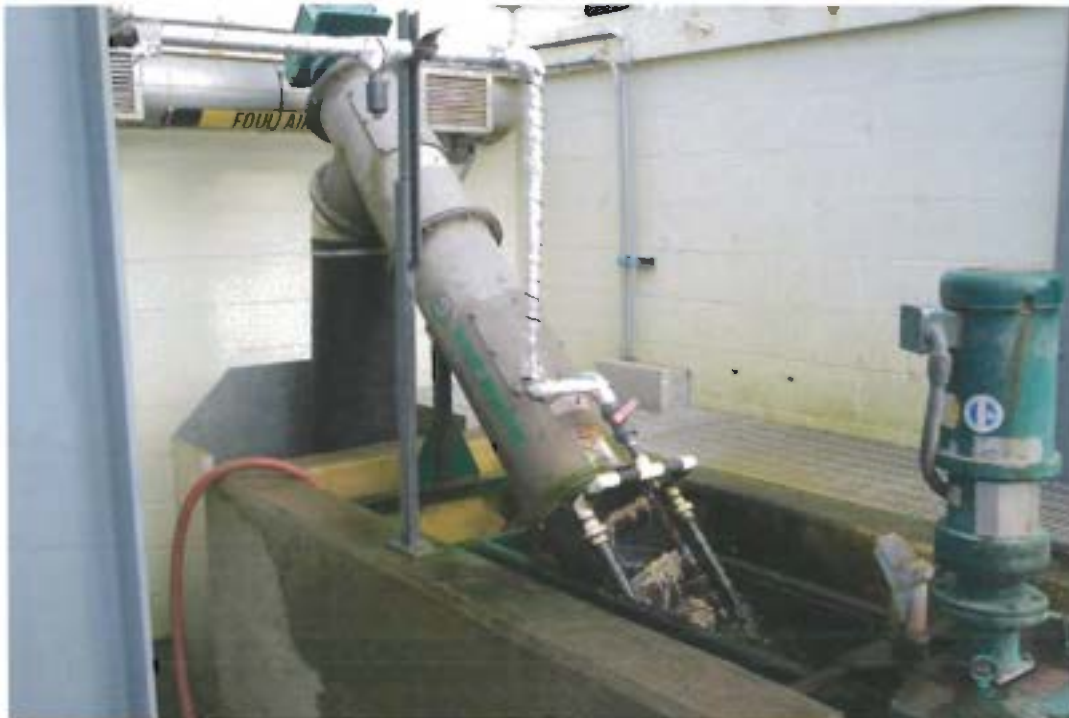
Headworks of Bandon WWTP
