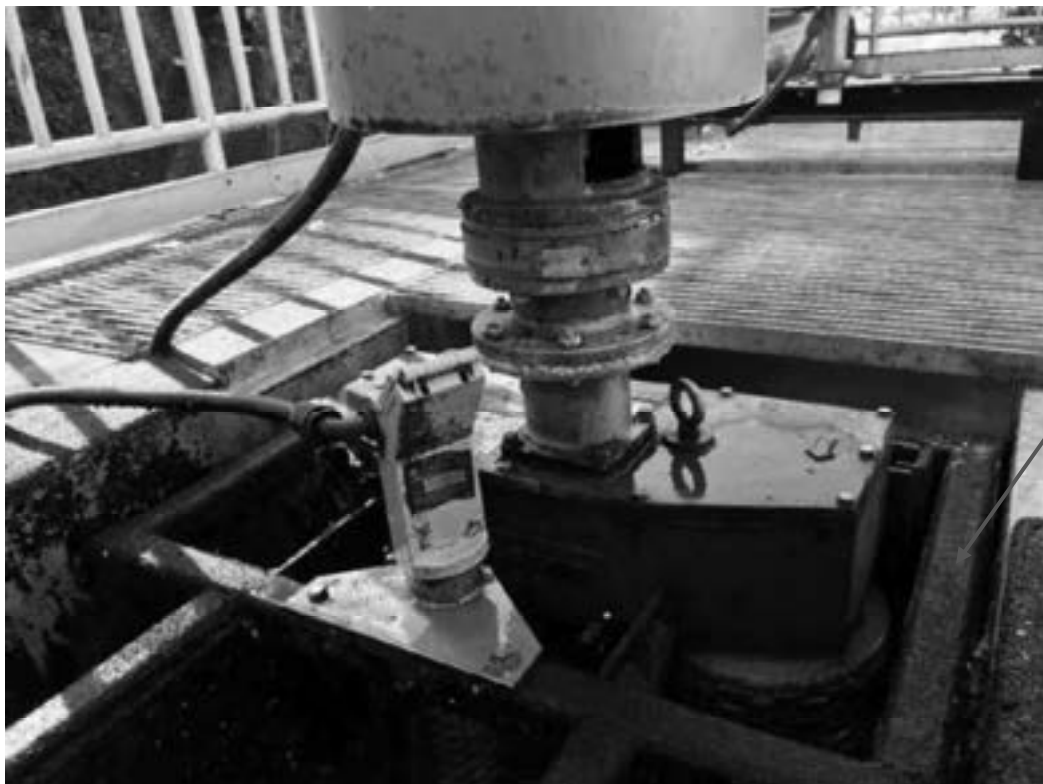
Grinder support structure showing moderate corrosion
