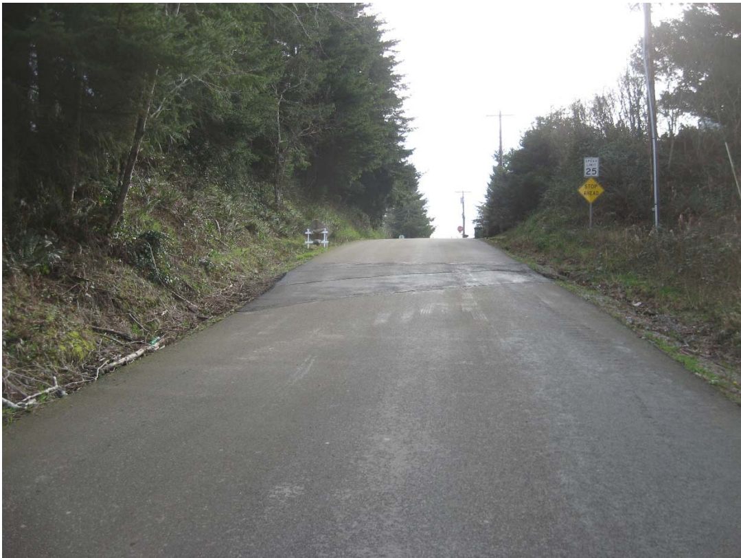
Photo 1. Offset on road pavement
