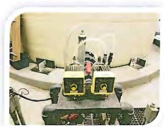
FIGURE 5.3.6 CHLORINE DOSING PUMPS
