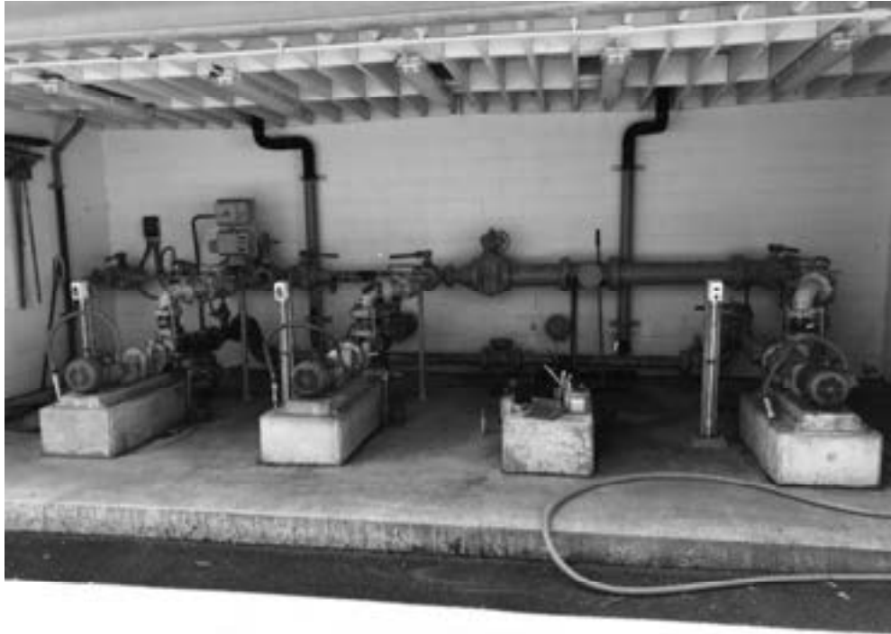
RAS/WAS Pump Area
