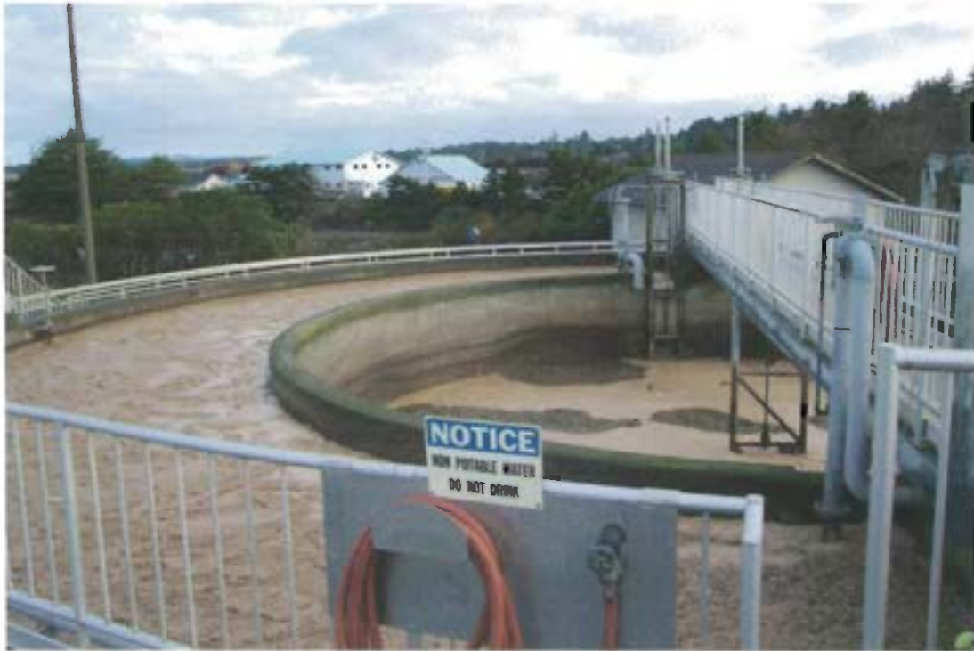
Bandon WWTP Digester
