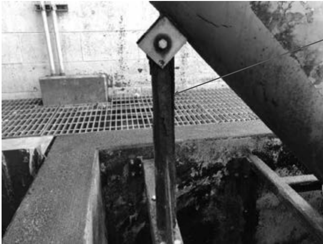
Screen support structure showing delamination of metal indicating severe corrosion.
