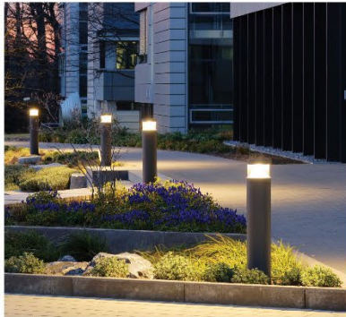
BOLLARD STREET LIGHTING
